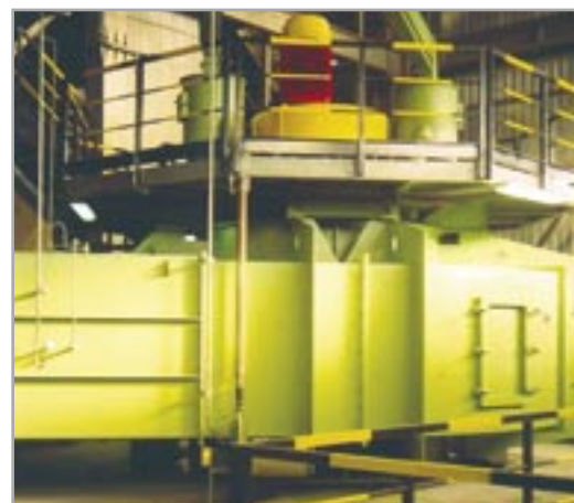
Air separator VTP 2900 at the cement grinding plant with a capacity of 130t/h – Galatina, Italy
