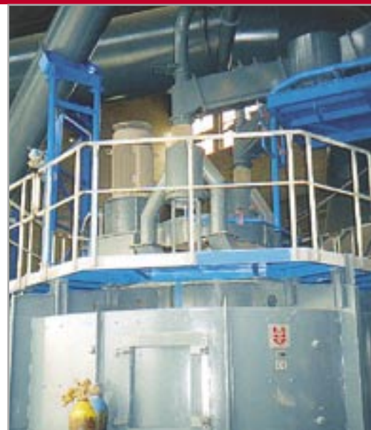
Air separator VTP 2400 at the cement grinding plant with a capacity of 72 t/h – Lukavac, Bosnia and Herzegovina
