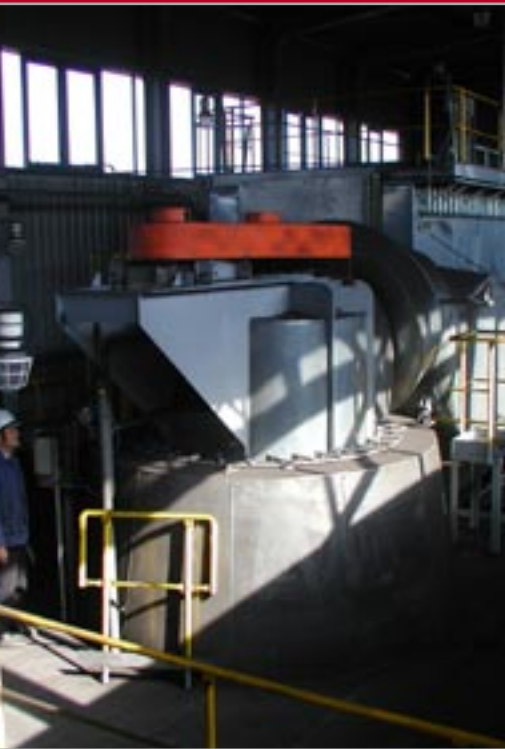
Air separator LTR-R 1650 at a coke grinding plant with 12.5t/h capacity – OKD Ostrava, Czech Republic
