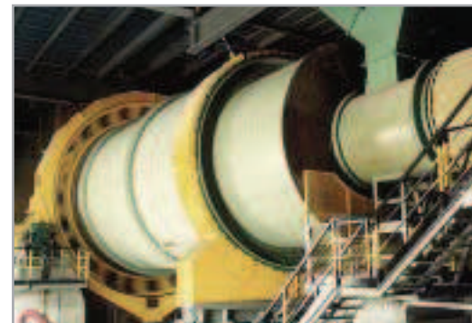
Raw mill Ø 5.4 x 11 m with a pre-drying chamber
