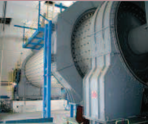
Cement grinding plant with a \varnothing 4.0 x 13.75 m mill seated on shoe-type bearings
