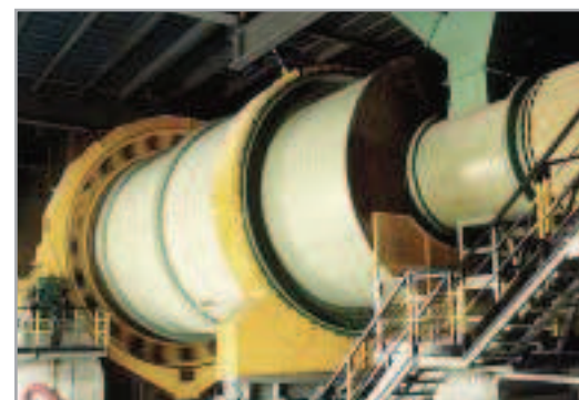
Raw mill Ø 5.4 x 11 m with a pre-drying chamber
