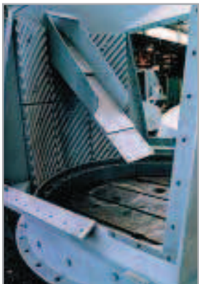
Armoring of the grinding chamber
