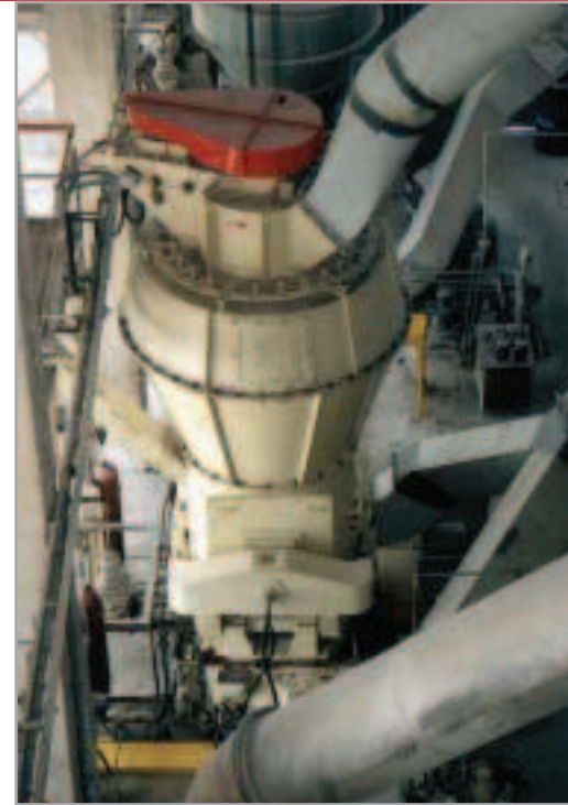
Dolomite grinding plant with a KTM 1200
